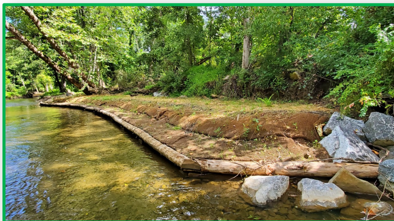
Modified Mud Sill used on the Frankstown Branch of the Juniata River to Stabilize the Streambank and Provide Aquatic Habitat
